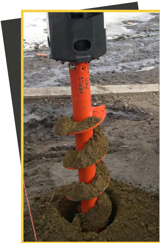
Pictured Left TriMax® Auger with 37 Gage and 5T30 Fas-N-Lok® Teeth drilling in frozen soil.
